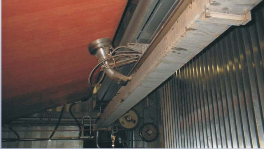
SUPER CLEANER INSTALLED IN PAPER MILL
